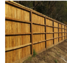
4.0m High BSW Warior acoustic barrier fence as specified in mitigation for background garden noise
